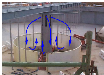
Existing simple Influent Column in the 55E Solids-Liquid Separation Tanks
